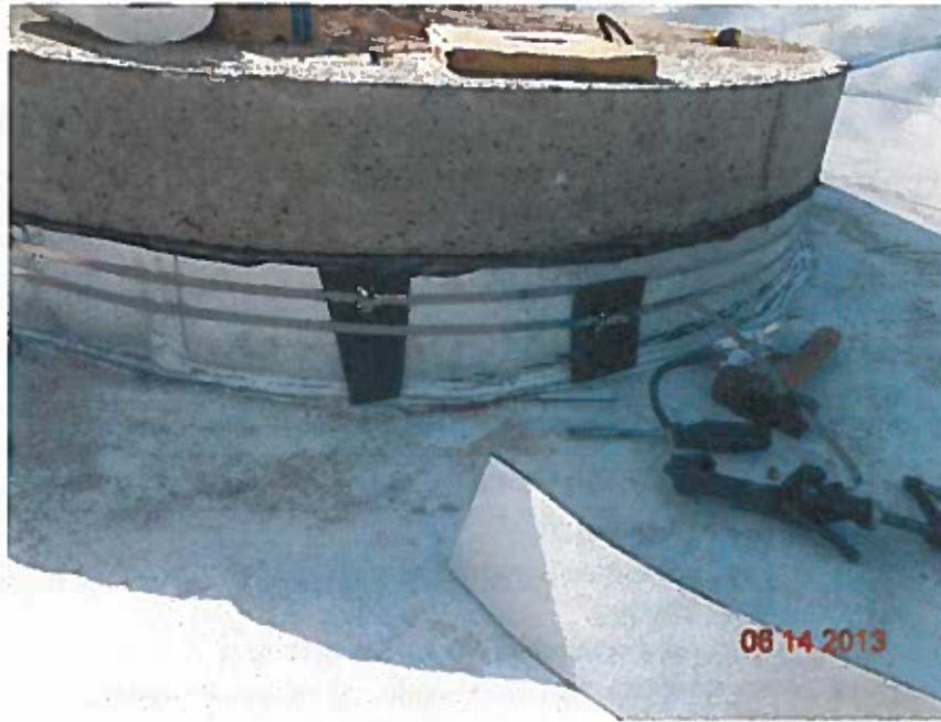
Basin overflow/discharge structure liner attachment – two offset clamps used, extrusion weld (spark tested)
