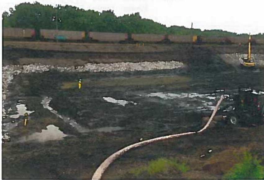
Northeast view of benched northern slope, northern access point, 6" dewatering pump, and southern access point at the Secondary Ash Settling Basin, facing northeast.
