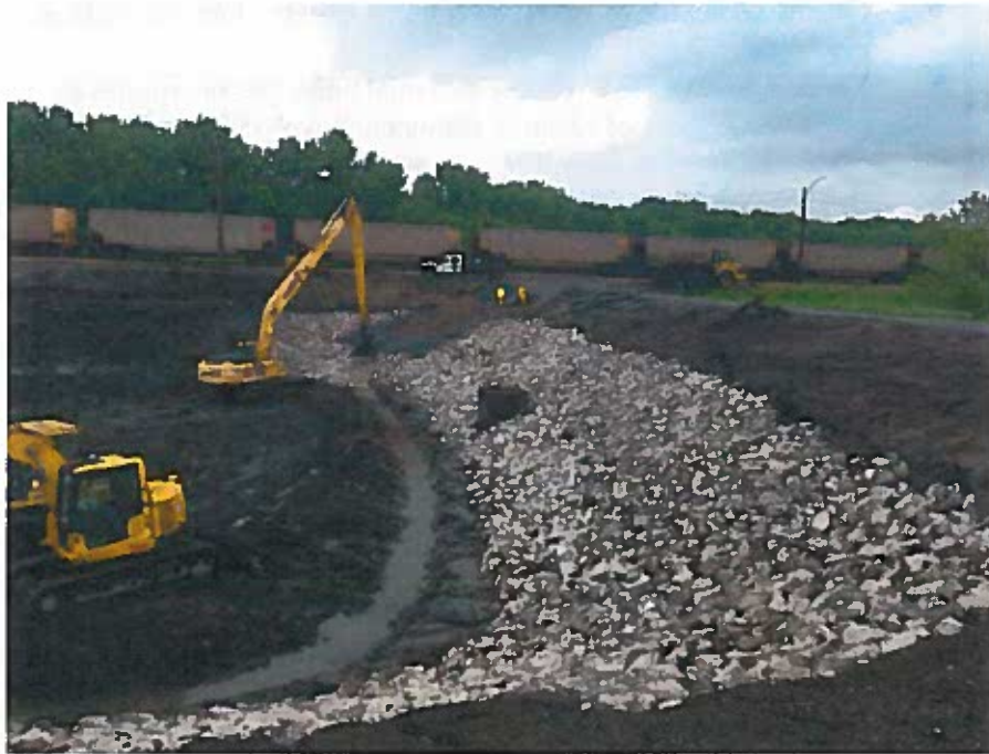
Northern view of: construction of access ramp at northeastern corner of basin; riprap stabilization layer one east slope; and beginnings of slope base drainage trench along eastern and southern slopes
