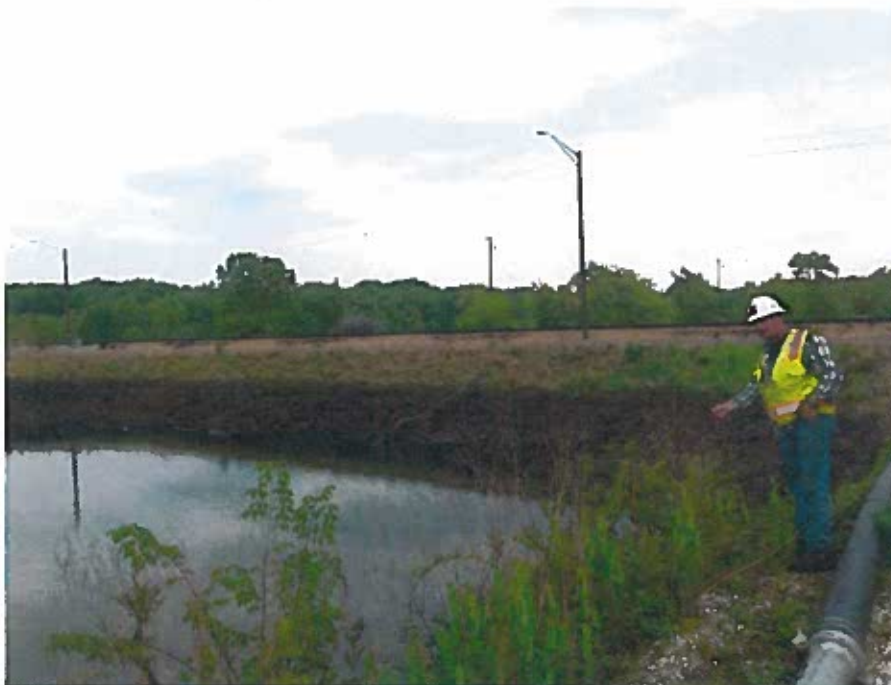
Northwestern view of high water mark on northern slope of Old Intake Channel, west of Secondary Ash Settling Basin
