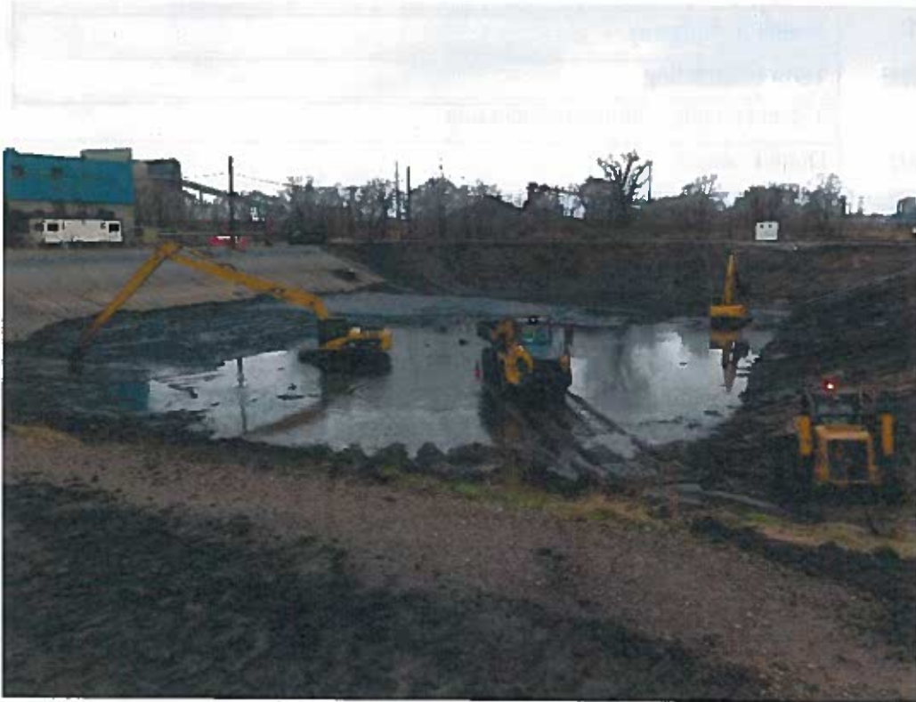
Southwest-facing view of: excavation activities with long-stick loading off-road truck in center; smaller excavator pushing material towards 8" pump located in the northwest corner (top right); and skid steer assisting with miscellaneous tasks (bottom right)
