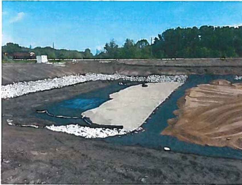
View of drainage layer progress on west side of basin with: subgrade, geotextile, and some drain tile on left; stone drainage layer in middle; and additional geotextile layer and cushion material on right
